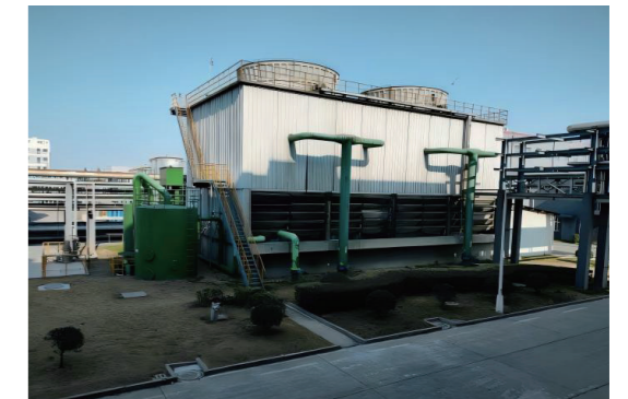
Water Recycling Facilities
